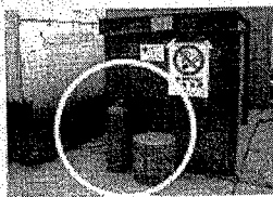
滅火器具 Fire fighting equipment
